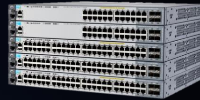
Existing deployments of HP switch ports
